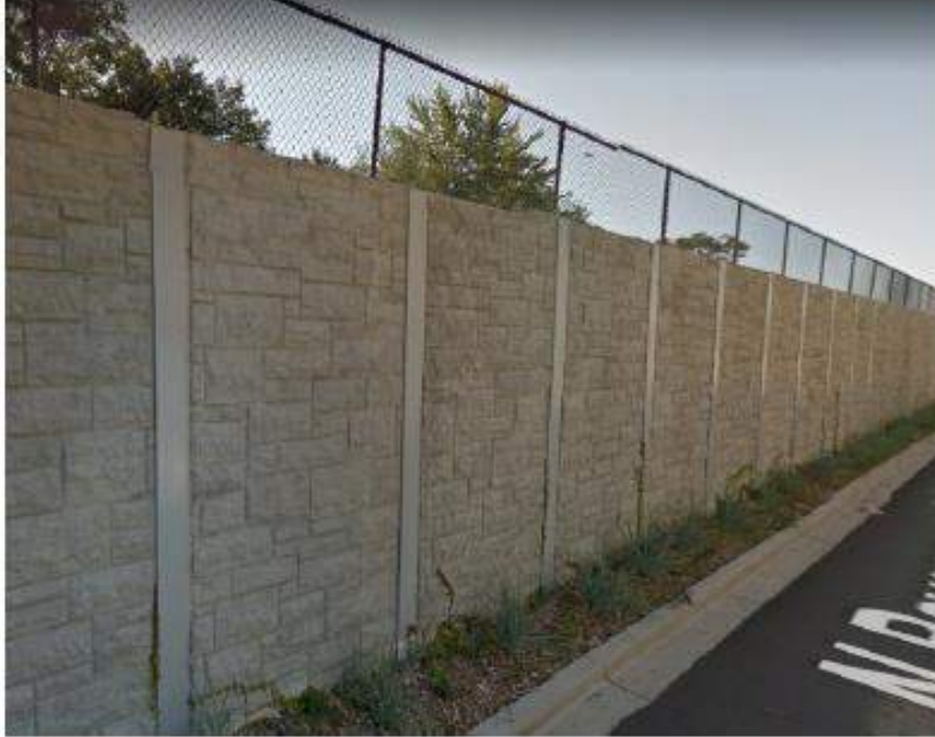
Figure 2-2: A Soldier Pile Retaining Wall Constructed for the Previous Grace to Balmoral Project
