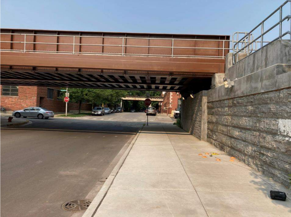
Figure A-22: Site STV-1, W. Berteau Ave. Metra Bridge, looking west toward Metra tracks
