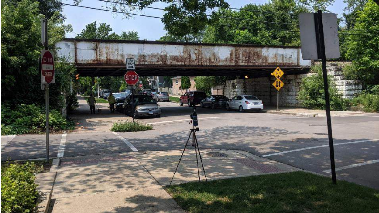
Figure A-14: Site STN-3, W. W. Barry Ave. Metra Bridge, looking west toward Metra tracks
