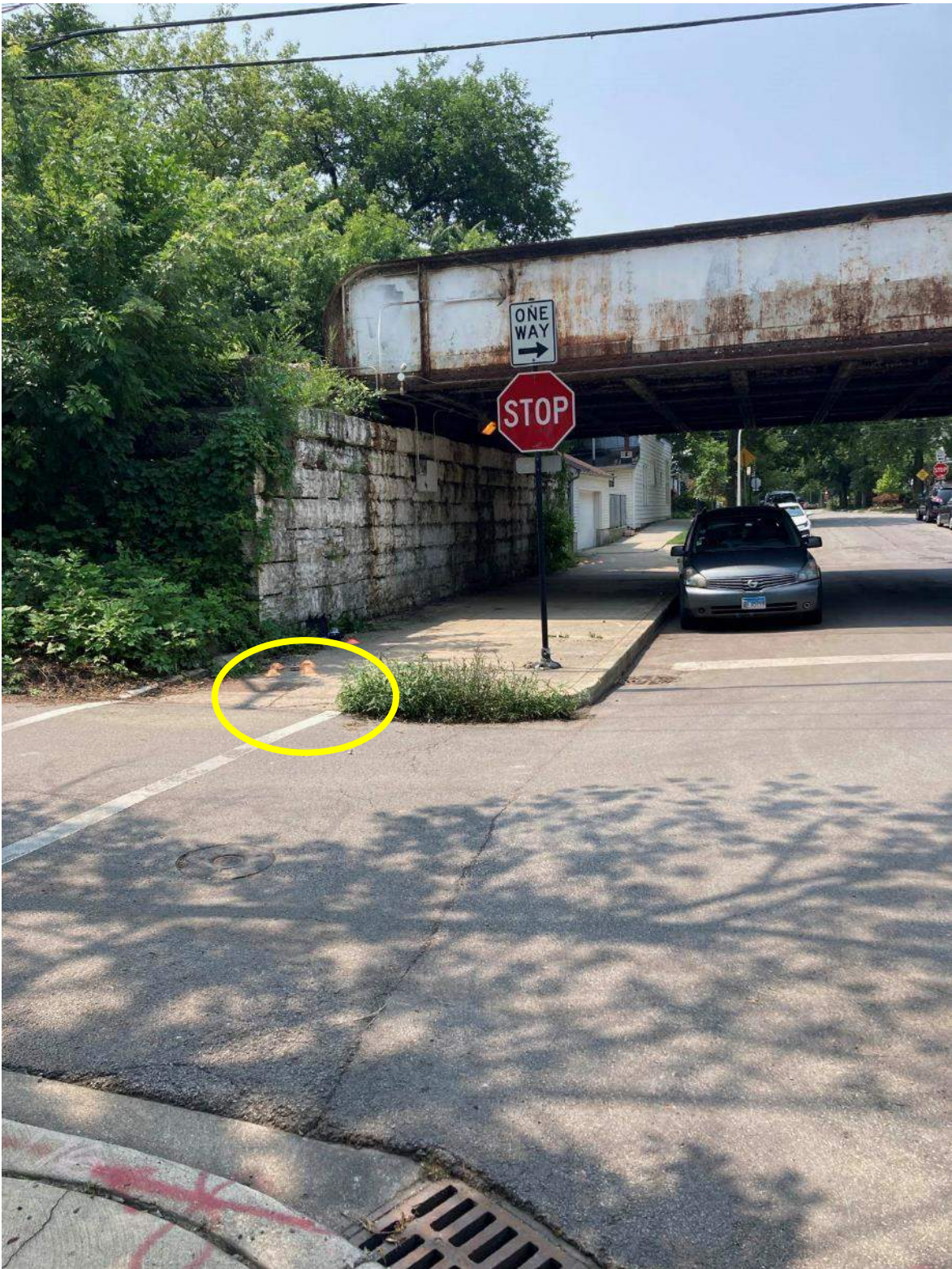
Figure A-24: Site STV-3, W. Barry Ave. Metra Bridge, looking west toward Metra tracks
