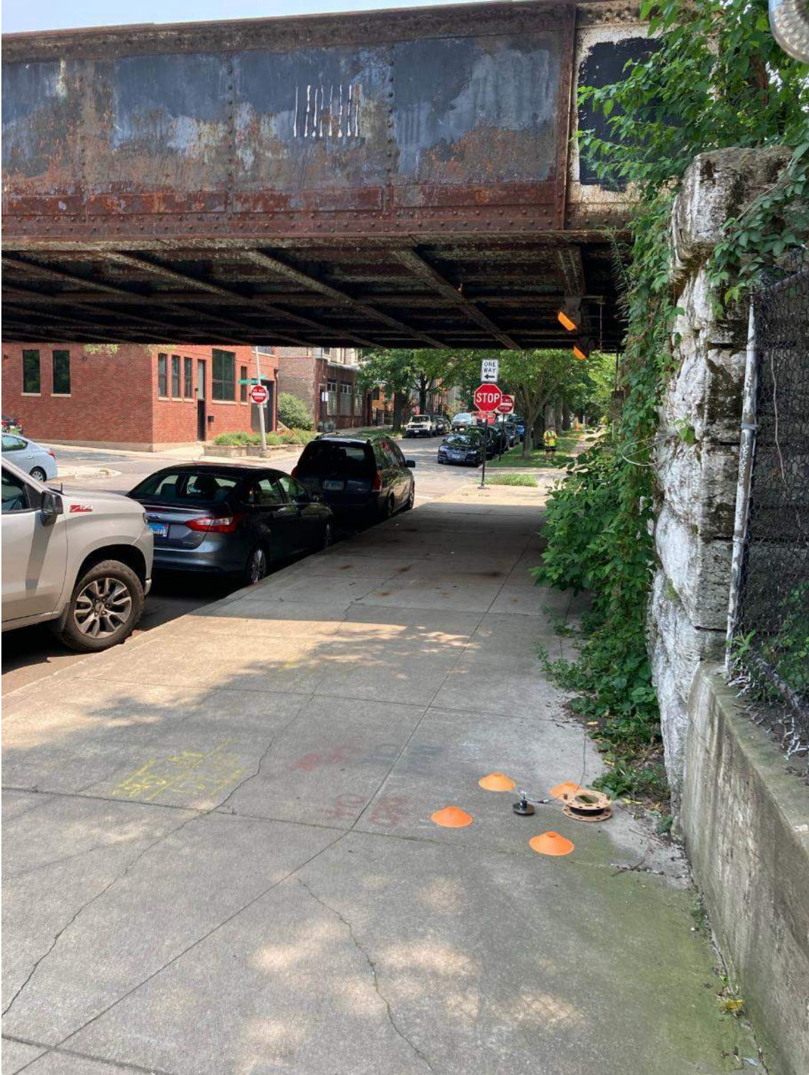
Figure A-25: Site STV-4, W. Barry Ave. Metra Bridge, looking east toward Metra tracks
