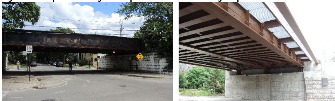
(Left) Existing bridge at School Street to be replaced; (Right) example of new bridge construction from UP North Line Grace to Balmoral Project.
