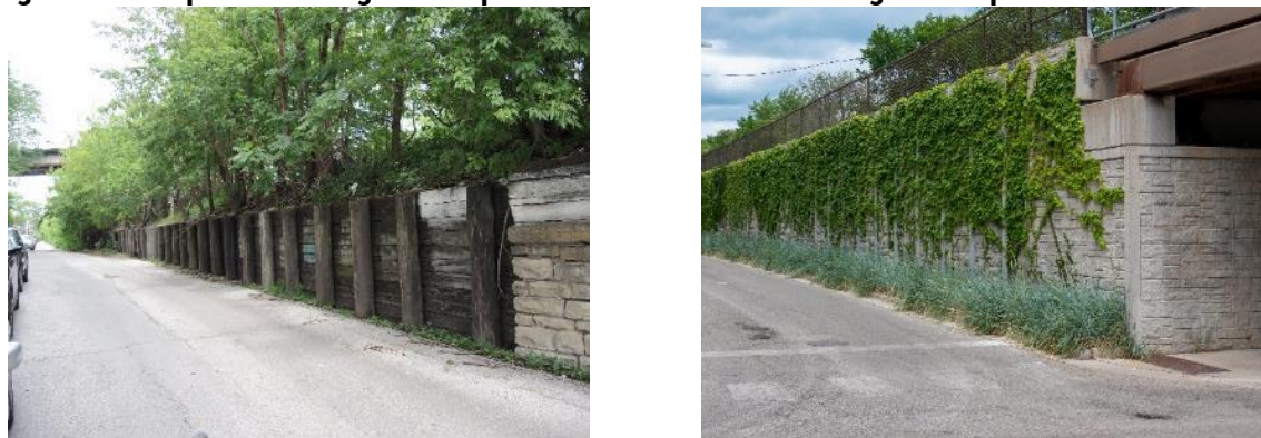
(Left) Existing retaining walls to be replaced along Ravenswood Avenue north of Roscoe Street; (Right) example of recently replaced retaining walls along Ravenswood Avenue from the UP North Line Grace to Balmoral Project.
