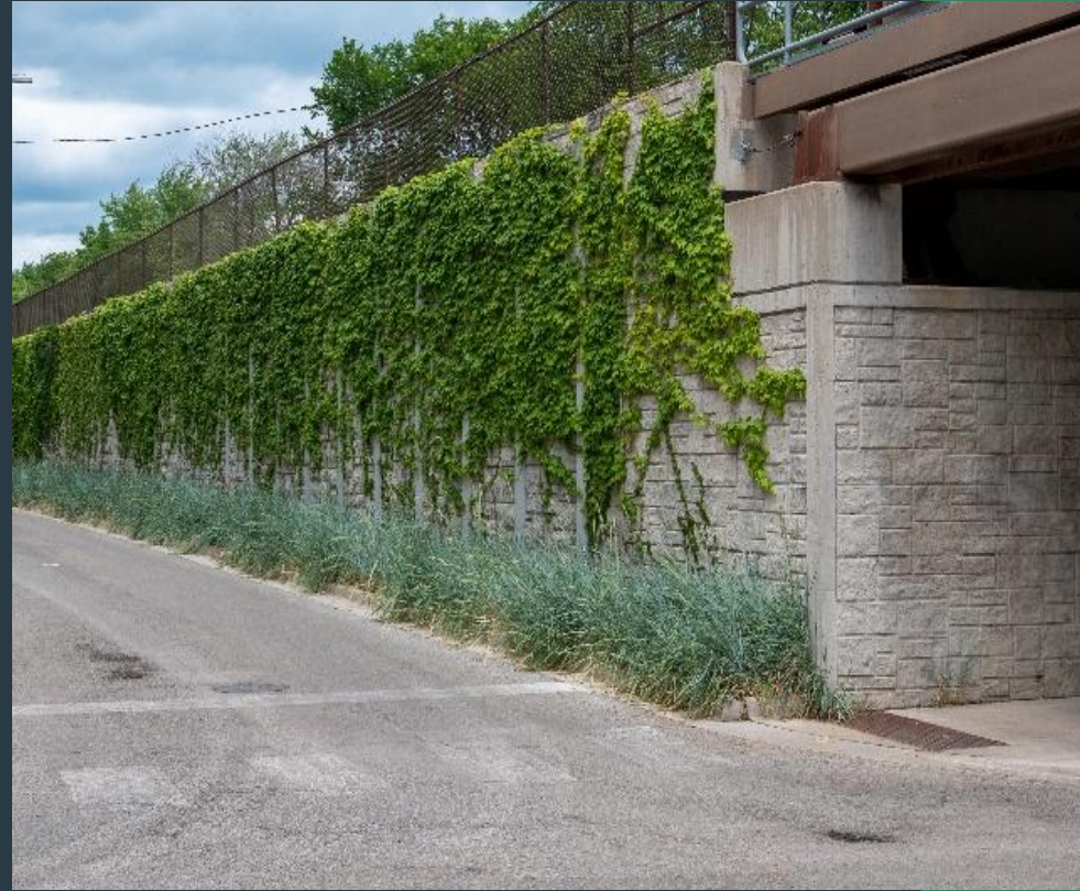
Recently constructed retaining walls along Ravenswood Avenue as part of the UP North Grace to Balmoral Project.
