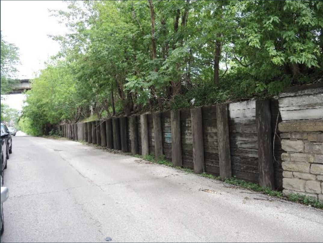
Existing retaining walls to be replaced along Ravenswood Avenue, just north of Roscoe Street.
