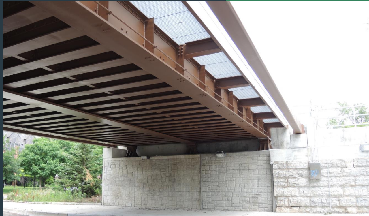
Example of new bridge construction from the UP-North Grace to Balmoral Project
